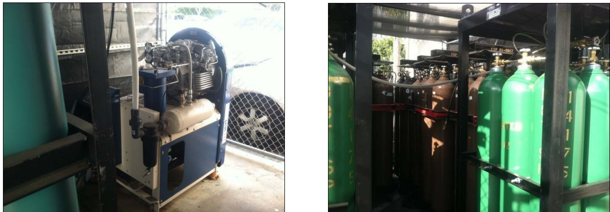
Figure 3 (left) High pressure compressor (right) "Dirty" helium storage in cylinders
